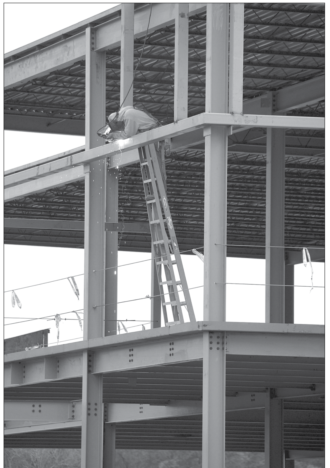
Photo contributed Work has begun on a 40,000 square foot New Hanover Regional Medical Center building in the Villages at Brunswick Forest, one of the area's fastest growing communities.
